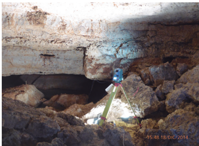
Figura 25. Hundimientos de techo en zona D4-D6. Figure 25. Roof subsidence in zone D4-D6.
